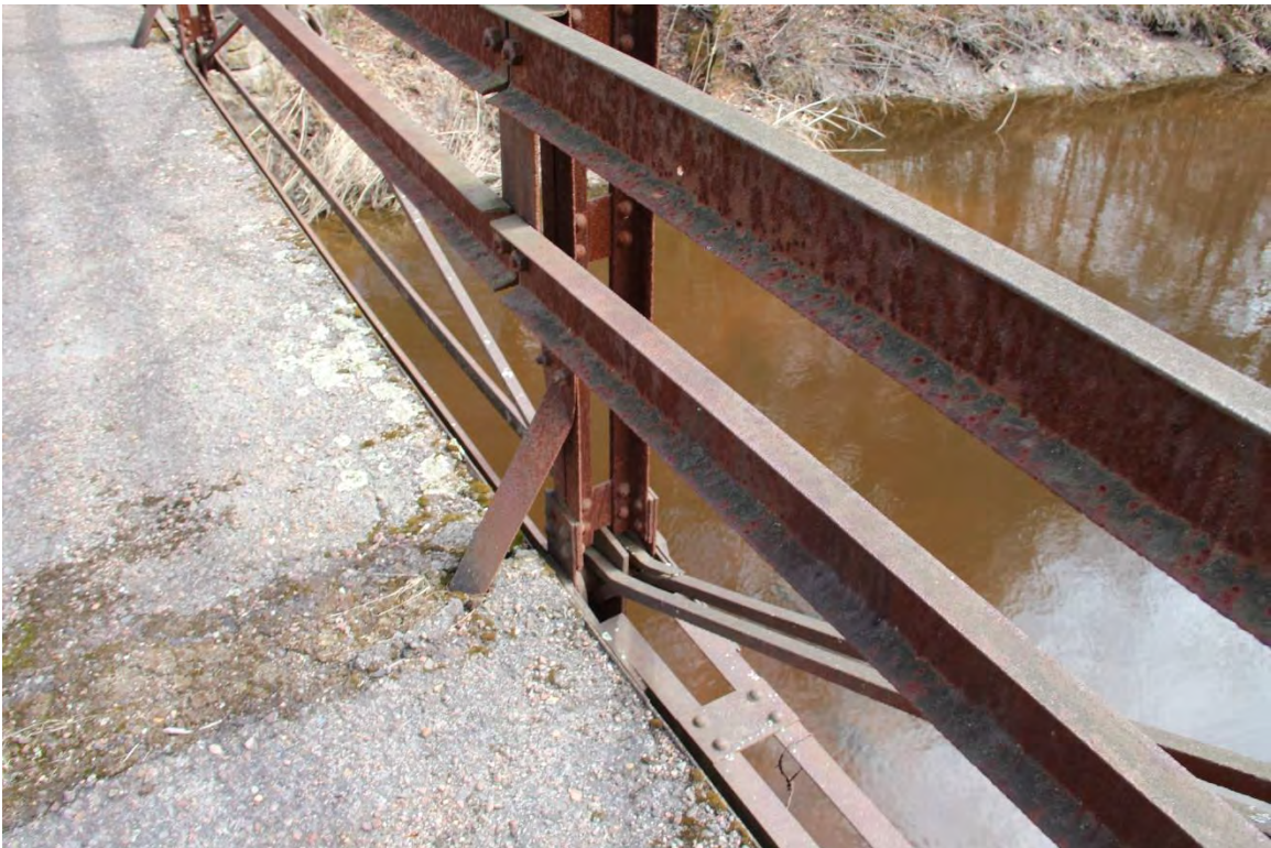
Photograph 4 of 11. Detail of bottom chord, vertical and diagonal members, and pin connection.
