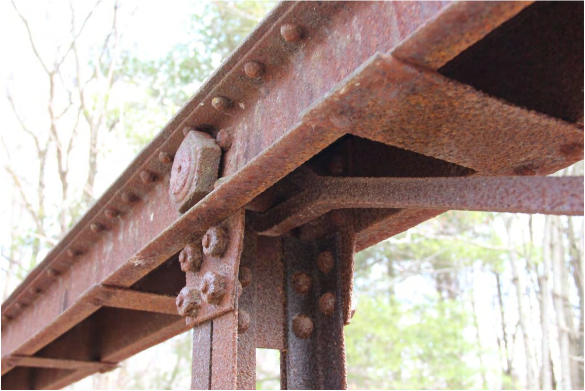
Photograph 3 of 11. Detail of top chord, major pin connection, and riveted and bolted members.
