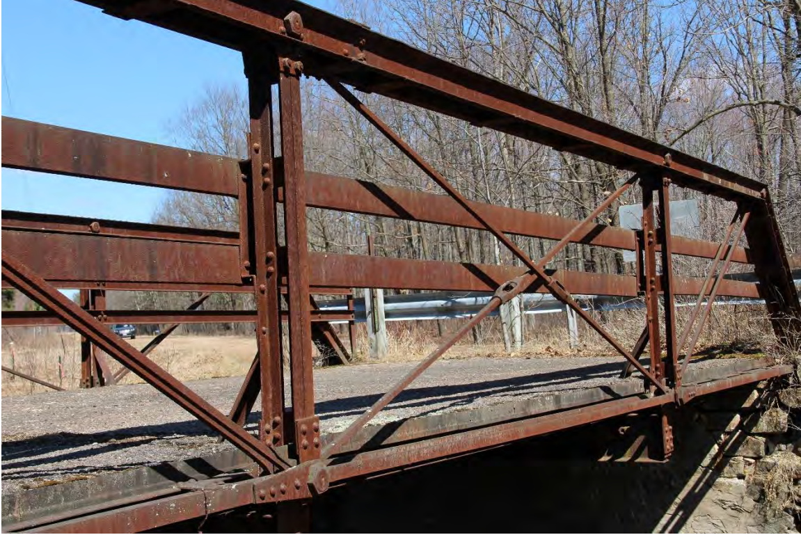
Photograph 5 of 11. Detail of central truss panel on southeast elevation, view facing north.
