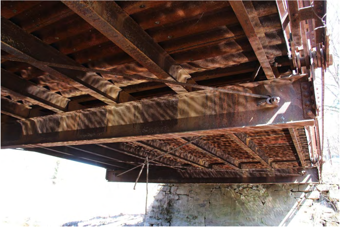
Photograph 7 of 11. Floor system with rolled I-beam stringers, floorbeams, and lateral bracing, view facing north.
